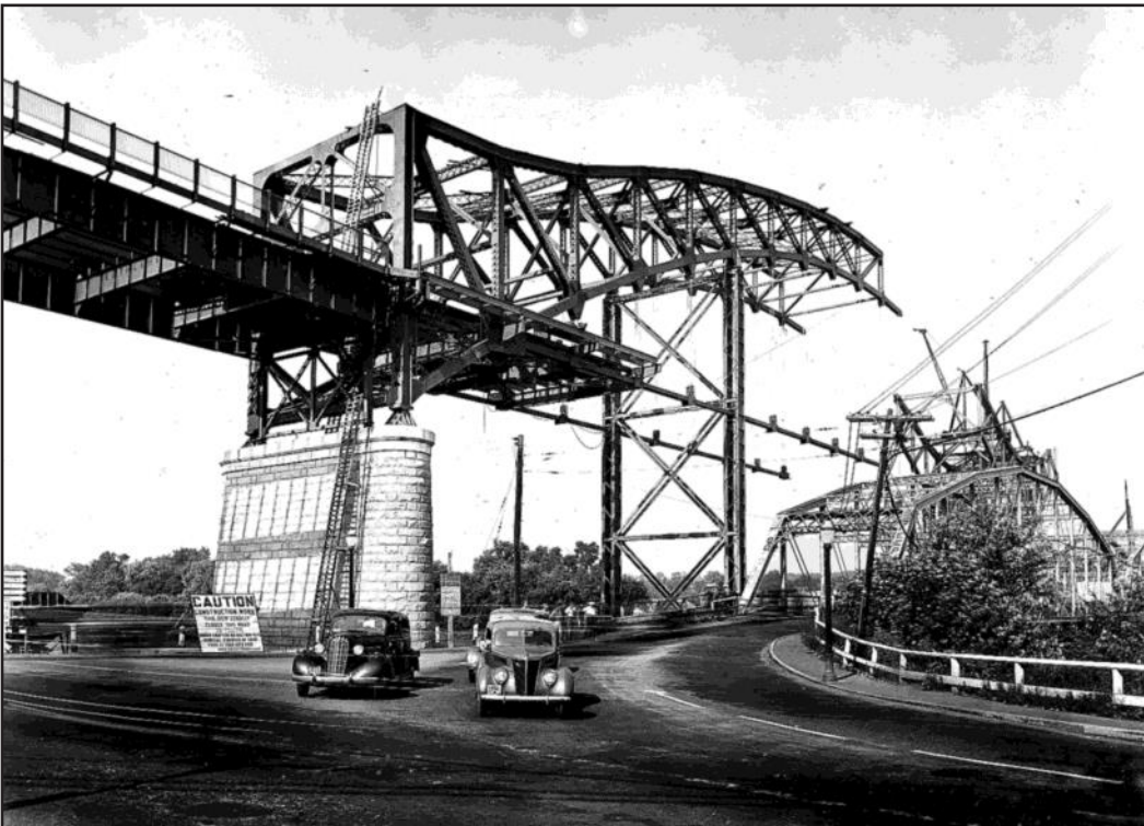
This photo, taken during construction of the new Middletown-Portland Bridge in 1936-38, shows several cars coming off the 1896 bridge on the Middletown side of the river. The old bridge remained in service throughout construction.
