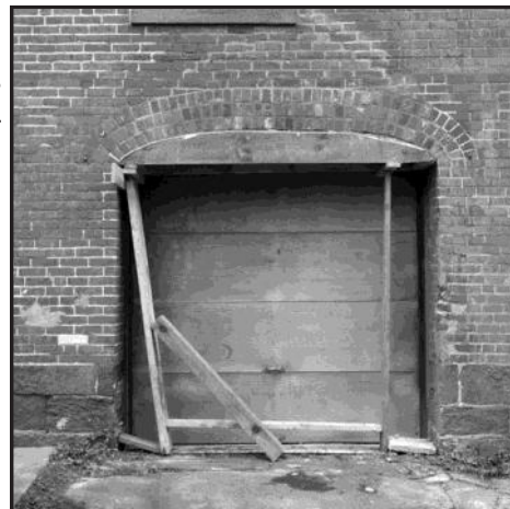
The ca. 1855 doorway on the north side of 646 Main Street--wide enough to accommodate wagons back in the day! The wooden piece going straight across the doorway forms a SUPPORT holding up the Basket Handle Arch above it, while it sets. This brickwork was done by Mark F. DeFrancesco. Photo by Kerry Heidenis (husband of Doris) at kerry.images@gmail.com
